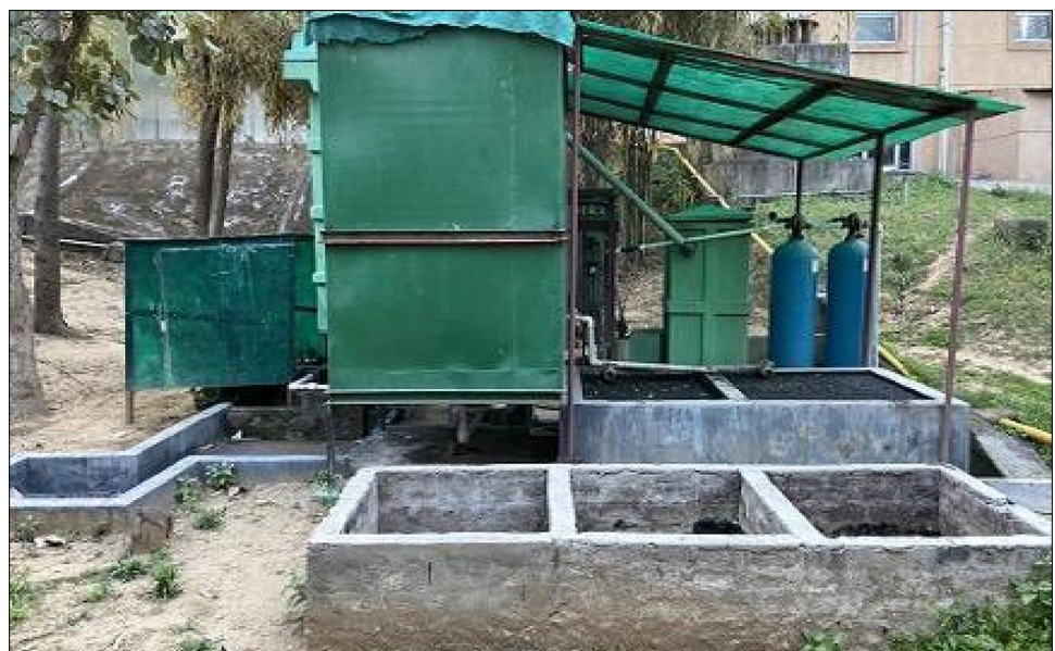
Fig. 1 Operating common sewage treatment plant (CSTP) based on MBBR at TERI campus
